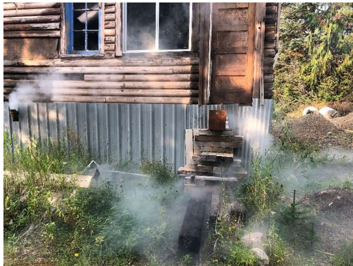
30651 E Meldrum St : Smoke billowing out of broken pipe / stub or other large opening in sanitary connections, old run-down house.
